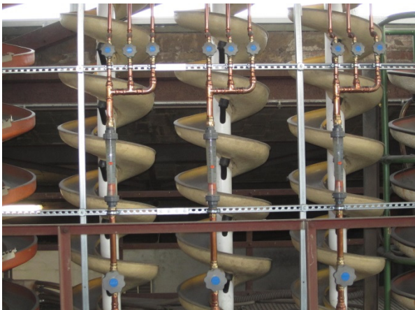
Rougher stage, consisting of 3 units spiral conc. type WW6PLUS, 7 turns.
