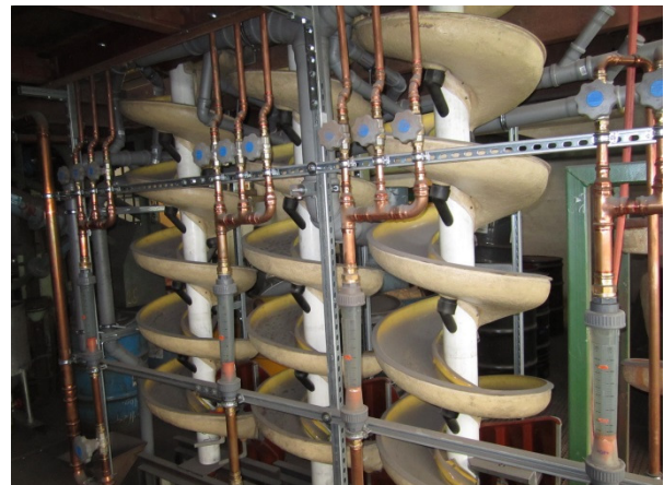
Cleaner stage 1, consisting of 3 units spiral conc. type WW6PLUS, 5 turns.
